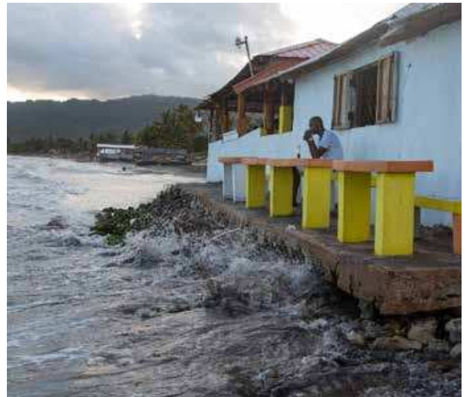
Erosion, storm surge and flooding threaten coastal restaurants, bars and homes, Alligator Pond, Jamaica. © Tim Calver
