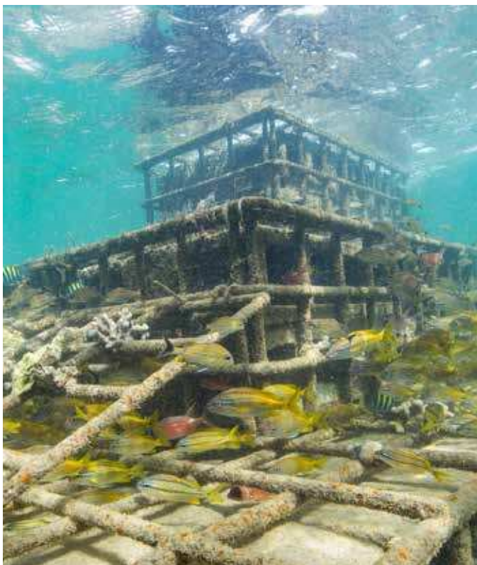
Pilot hybrid or 'artificial' reef structures, built with steel cages and filled with stones and cement, to protect a vulnerable coastline from strong wave action and the impacts from climate change, such as severe erosion © Tim Calver
