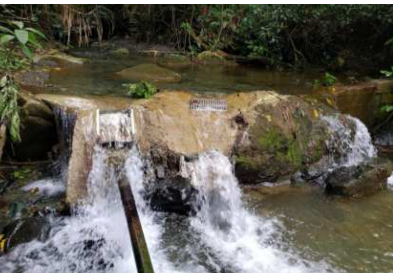
Illustration 13: Example of surface catchment in the Las Piedras gravity flow water supply systems in San José de las Matas. Source: SIASAR.
