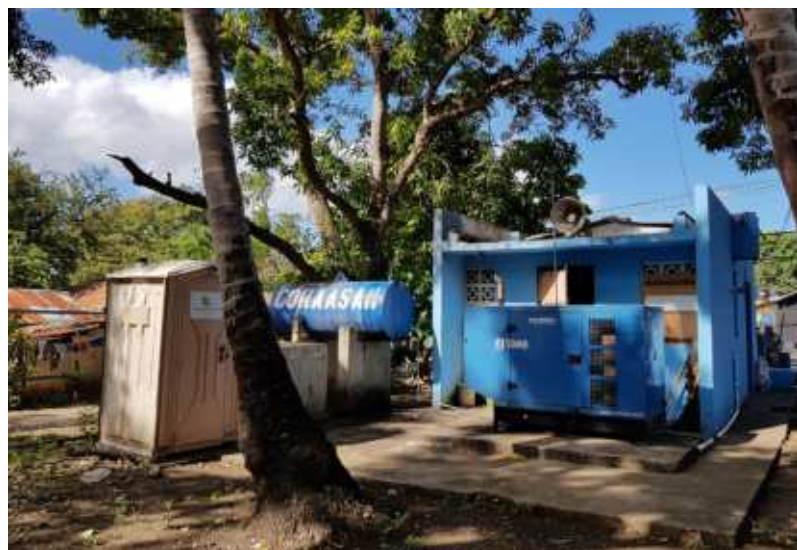
Illustration 14: Example of underground catchment by electric pumping managed by CORAASAN in Los Cocos, municipality of Santiago de los Caballeros. Source: Authors' preparation.
