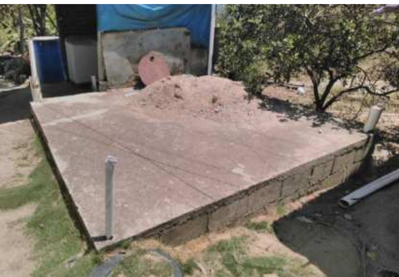
Illustration 11: Construction of a new installation over a pit. Source: CORAASAN household survey.
