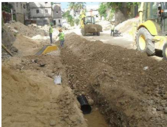
Photo 3-2: HDPE Pipeline installed in Phase I of the Project, similar to those to be used in Phase II
