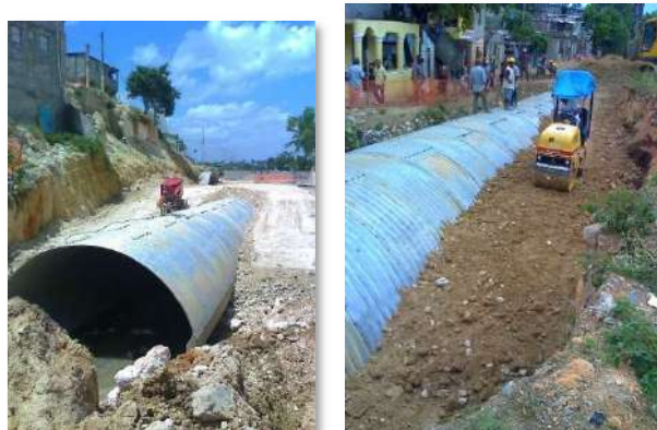
Photo 3-1: Metal Pipes installed in Phase I of the Project, like those to be used in Phase II.
