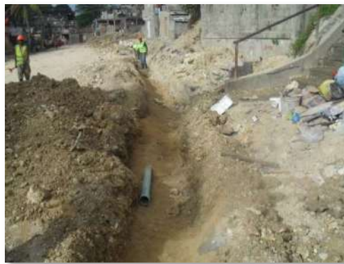
Photo 4-7: Pipeline for Water Supply in Phase I of the Project
