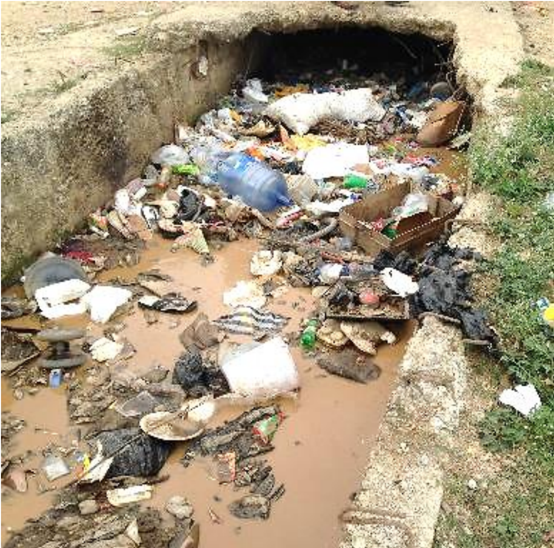
Figure 5.1: Solid Waste Accumulation in Channelized Creek in La Zurza
