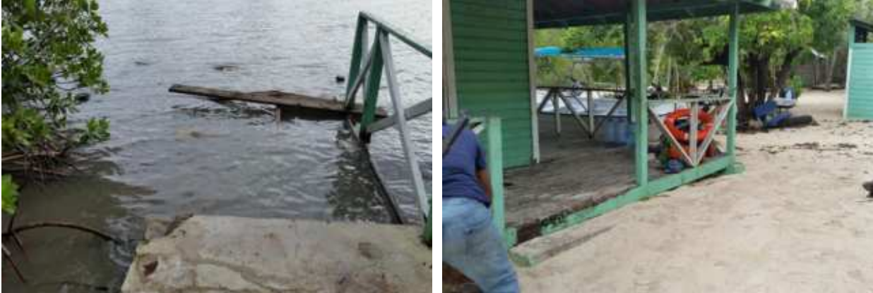
Photo 6. Damage from Hurricane Irma to infrastructure of the Marine Mammal Sanctuary of Estero Hondo, September 7, 2017.
