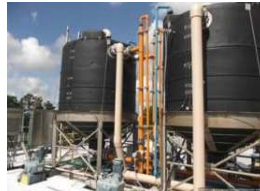
Figure 16. Chemical tanks with proper hold down straps
