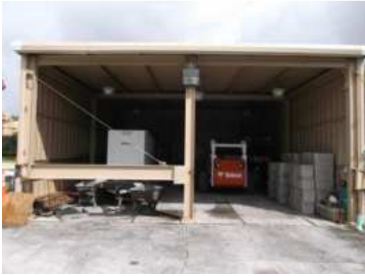
Figure 4. Open metal structure- recommend enclosing structure to reduce failure potential
