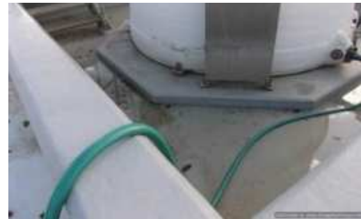
Figure 14. Chemical tanks with proper anchor
