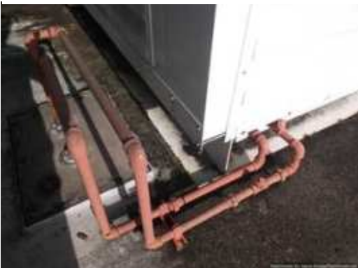
Figure 17. Lack of anchor bolts on generator
