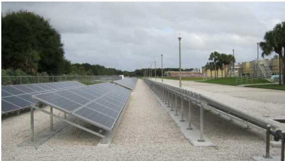
Figure 3. 184 KW Solar System at Palm Beach County Water Reclamation Plant
