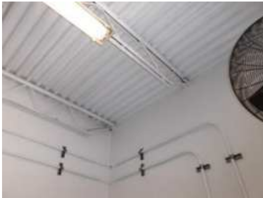
Figure 6. Roof joist to wall connection- recommend adding bracket to secure wall and roof
