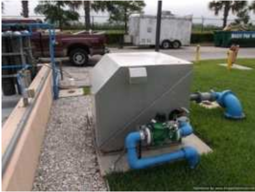
Figure 13. Equipment lacking tie-down
