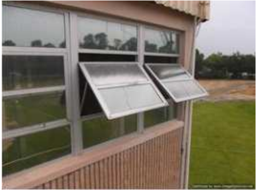
Figure 7. Unprotected window-recommend hurricane shutters or impacted rated windows
