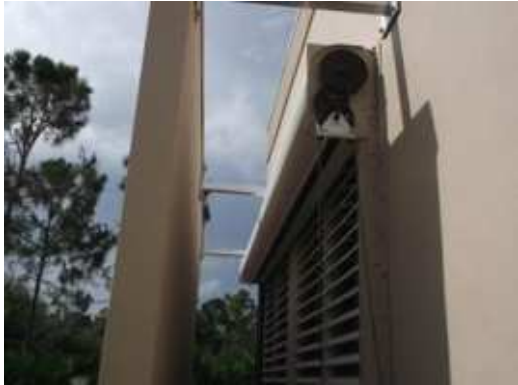
Figure 8. Wind wall installed to prevent wind driven rain from entering thru louvers
