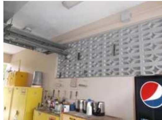
Figure 5. Unreinforced decorative wall block- recommend removal and replace with solid wall
