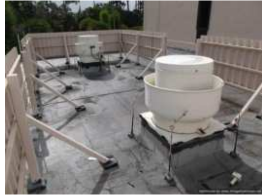
Figure 12. Tie down of roof equipment
