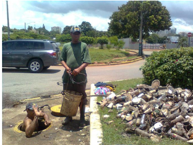
Figure 2: Workers unclogging storm water drainage systems in Santo Domingo, at Ciudad Universitaria, July, 2011.
