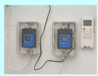
Controls for the humidity and other environmental parameters.
