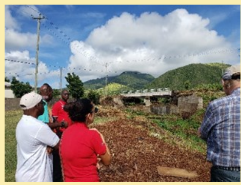
Viewing progress in works to rehabilitate the College Street Ghaut, St. Kitts, 18th October 2019.
