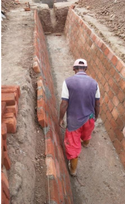
Photo 2. Trench lining process in preparation for the installation of a biodigester at the Julio Trigo Credit and Services Cooperative.
