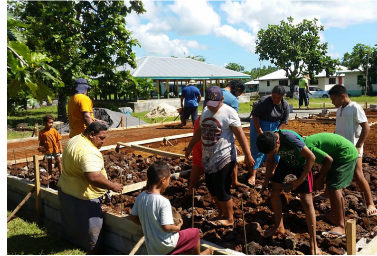
Residents of Setāfaō Saipiipi, Samoa, lay the foundation for a Seacology-funded community center.
