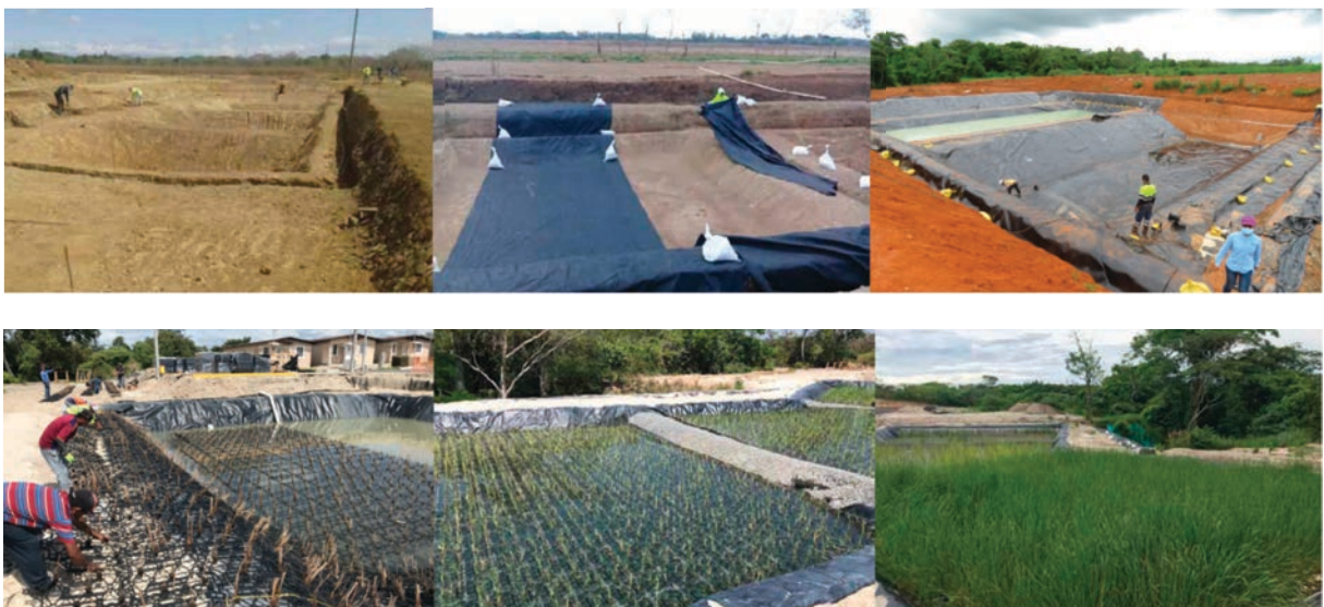
Figure 4: Overview of the individual construction steps. Earthworks, laying of the geotextile, installation of the watertight geomembrane as well as planting of macrophytes, commissioning and fully operational floating treatment wetland.
