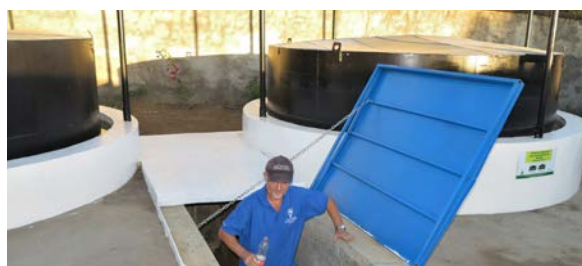
Figure 3: Service access to floating drum biogas reactor (T.18)
