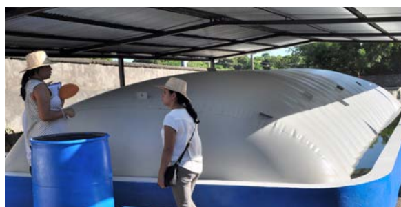
Figure 5: Anaerobic baffled reactor (T.3) with membrane cover
