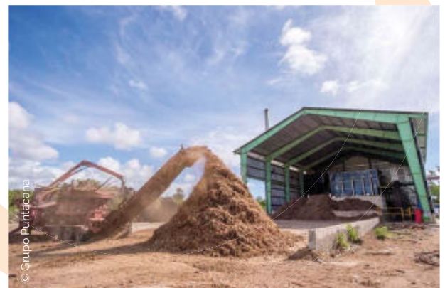
Biomass boiler, at Punta Cana Laundry Service.
