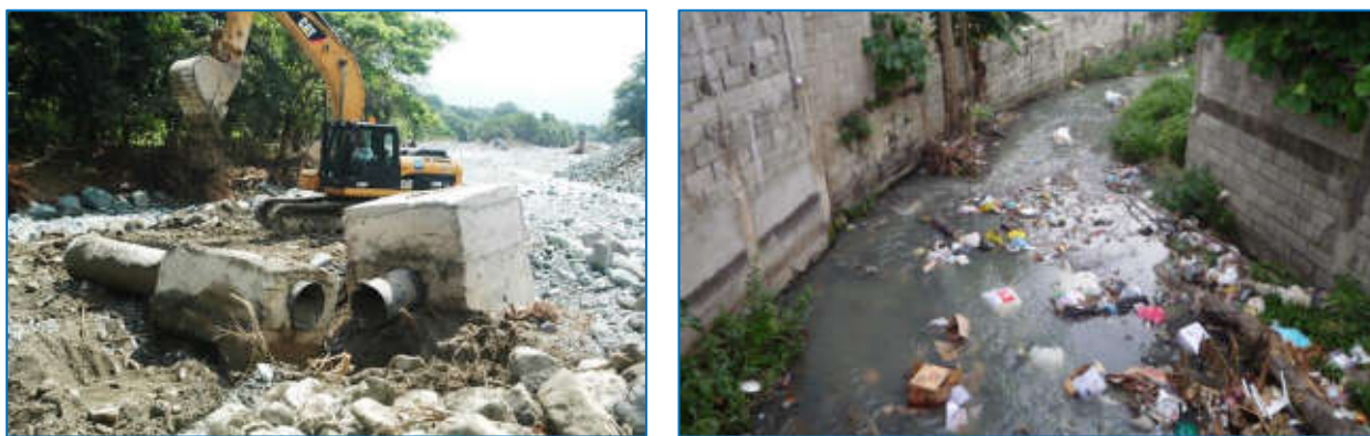
Figure 3: Water Sources Contamination in San Cristobal
