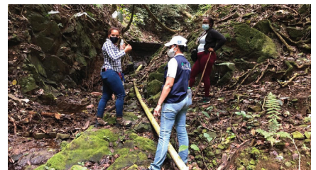
Water pumping test to measure flow provided to feed water storage tank being built for aqueduct of Loma Verde Community, one of several designed to supply water to rural areas.
