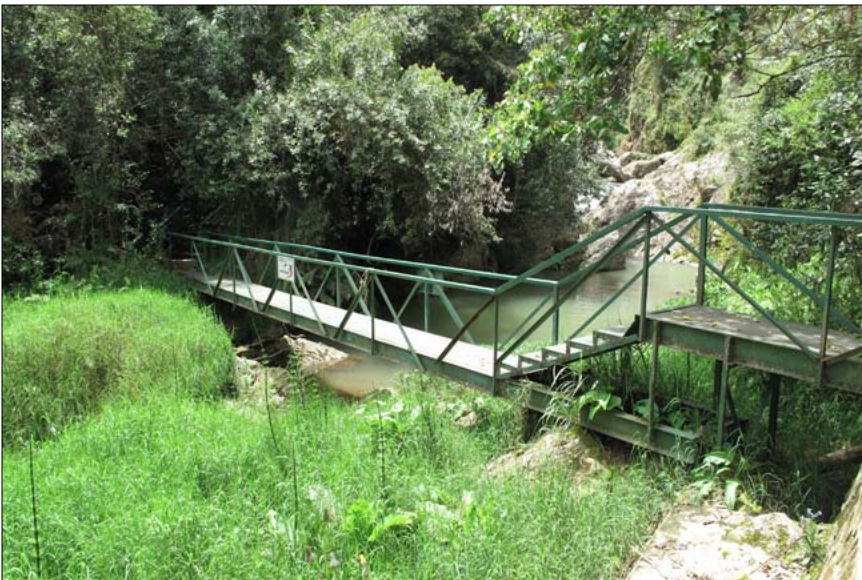
The metal footbridge and all metal railings have recently been repainted with blue paint.
