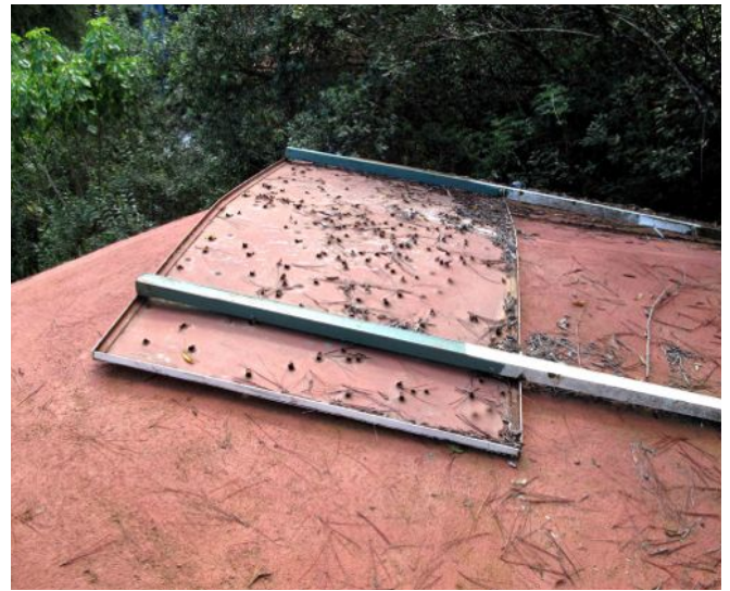
Photo 13. The large metal Brugal Rum sign atop the bathrooms should be removed.
