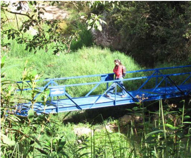
Photo 14. The recently painted metal bridge and handrails are already peeling. When repainted, the original green color is recommended.
