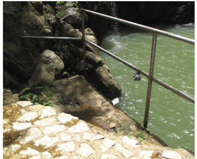
Photo 15. The platform and railing at the main observation platform are in need of immediate repair.
