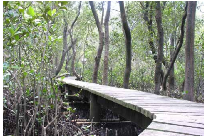
Photo 4 – Boardwalk trail without a hand rail.
