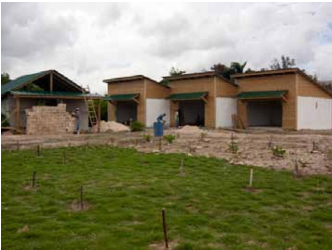
Photo 14 – The 3 partially constructed cement structures and a restroom facility (on left) are being finished.
