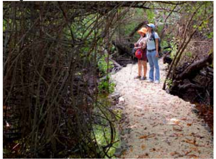
Photo 4 – The newly constructed trail from the office to the lagoon is constructed on the mangrove forest floor and covered with limestone rock.
