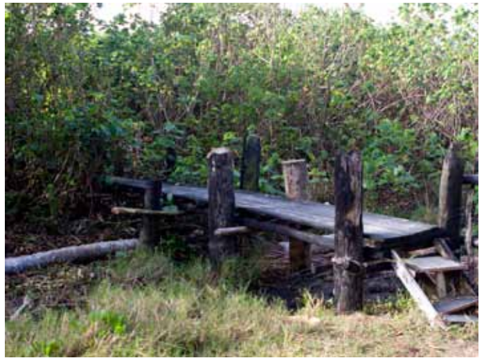
Photo 8. Boardwalk leading from Limón Beach to the lagoon. This is a safety hazard to visitors.
