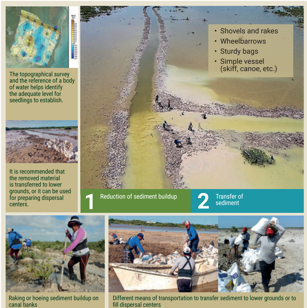
Figure 2.19 – Steps and recommendations for sediment removal for the topography rehabilitation in the mangrove ecological restoration. Prepared by Oscar Pérez, Andrés Canul and Diana J. Cisneros.
